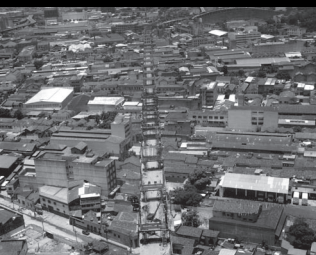
Fig. 1 1993. Aerial image from the construction of the elevated expressway on existing local roads of São Cristóvão. Department of Traffic and Transportation Management of the State Government of Rio de Janeiro.
